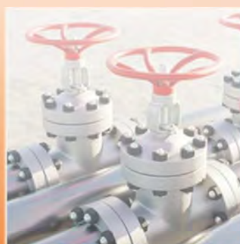
Natural Gas Pipeline
